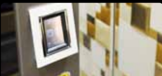
Touch screen device with home automation interface
